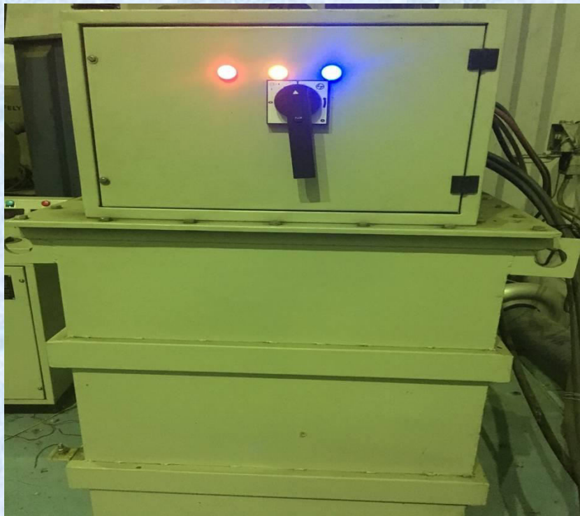
3-Phase Booster Transformer, 75 kVA, 2000 V & 52 Amps
